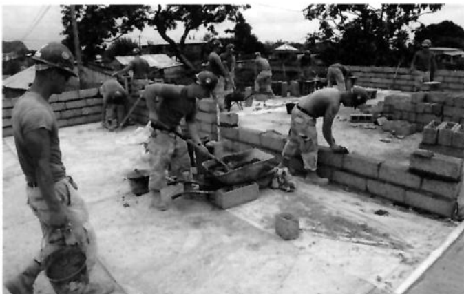
Seabee personnel construct a six-room schoolhouse in Maroni, Camoros, in support of the humanitarian assistance element of U.S. maritime strategy as set forth by the chiefs of the maritime services in 2007. (Kenneth Fidler)
